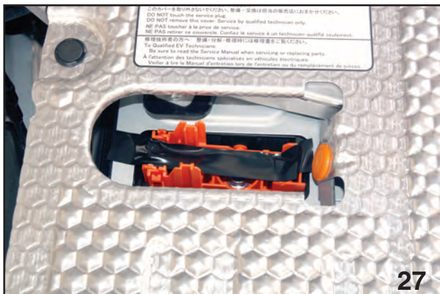
Electrical Tape over exposed terminal
