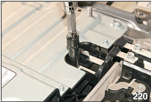
Positive and Negative High Voltage Battery Terminals
