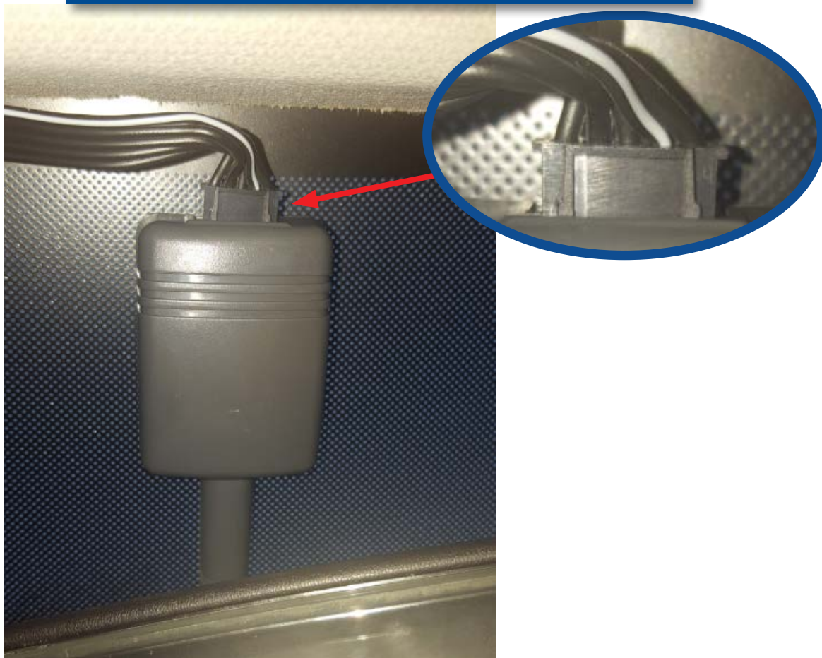
RES Antenna Connection – Not Secured
