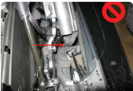
Incorrect position of the plastic water diverter
