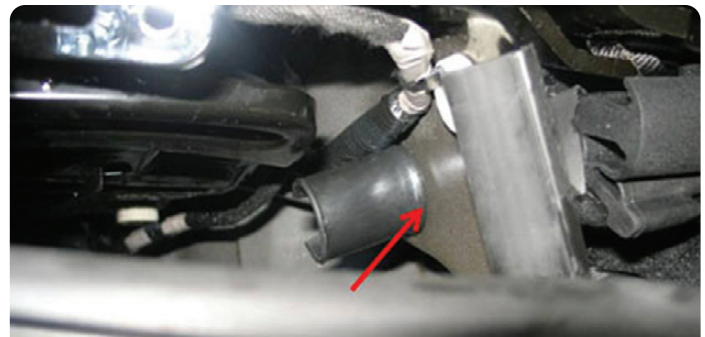
Front drain that is NOT fully seated in the sheet metal panel.
