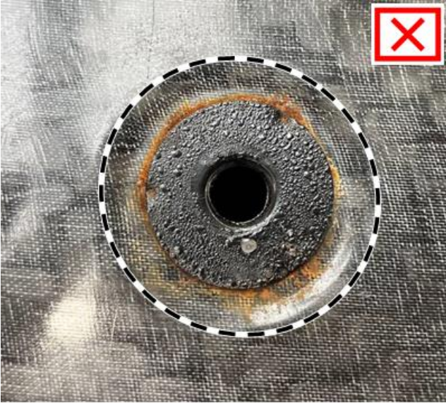
Figure 3 (areas are corroded = not OK)
