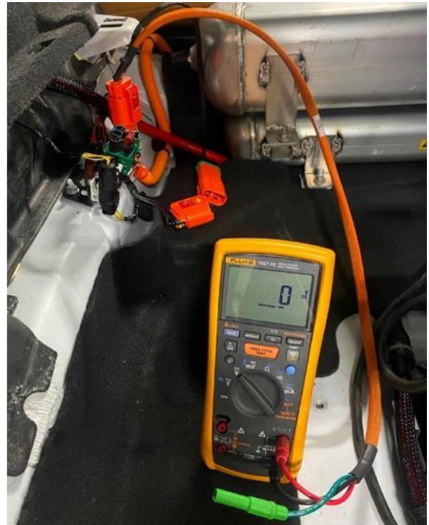
Figure 14 – PHEV Circuit Testing
