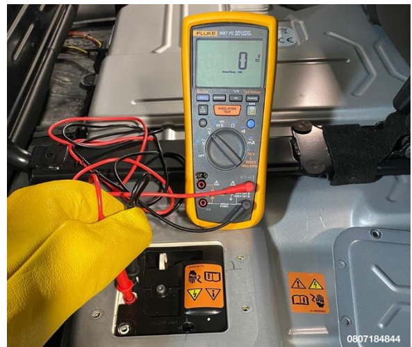
Figure 6 – Measuring at High Voltage Test Points
