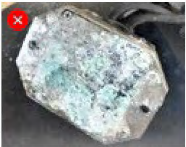
BACK SIDE COVERED BY CORROSION - REPLACE
