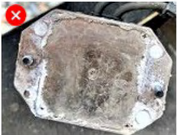
WHITE CORROSION ALL AROUND THE COVER - REPLACE
