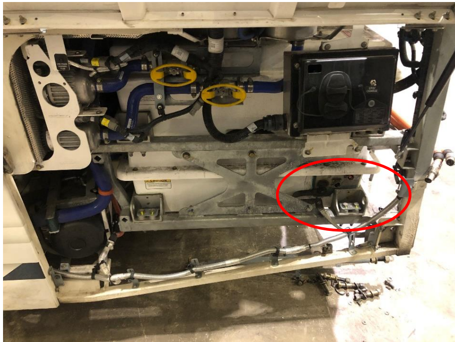
Figure 5: HV Connections and Ground Strap at Rear Street Side
