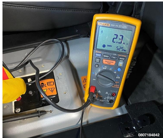
Figure 42 – Measure and Record Isolation Resistance Between HV Positive Test Point and Chassis Ground
