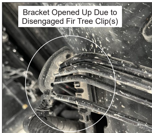
Figure 7 — Dodge Fuel Line Bracket Loose
