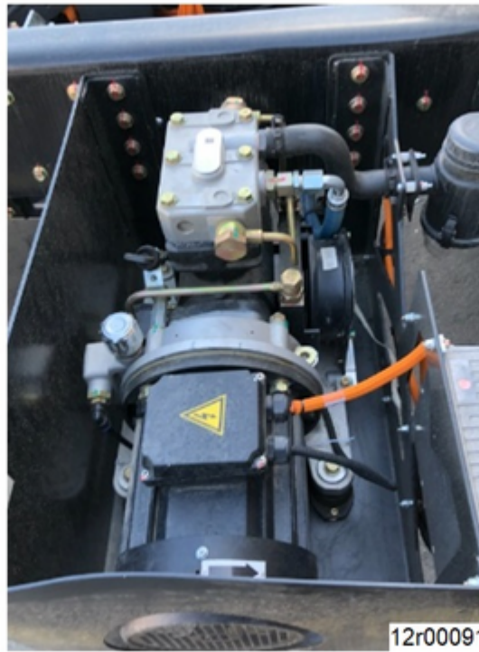
Figure 1, High Voltage Air Compressor Motor without Ground Strap (Action Required; see Resolution).
