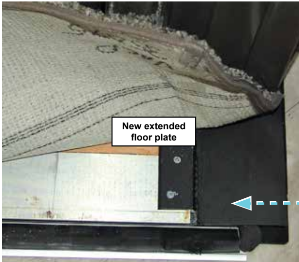
Figure 3-1 View of completed installation of new extended floor plate and new extended seal
