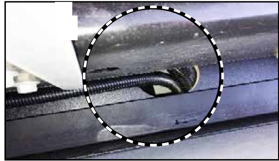
Figure 1-12 Example of hole near fuel tank
