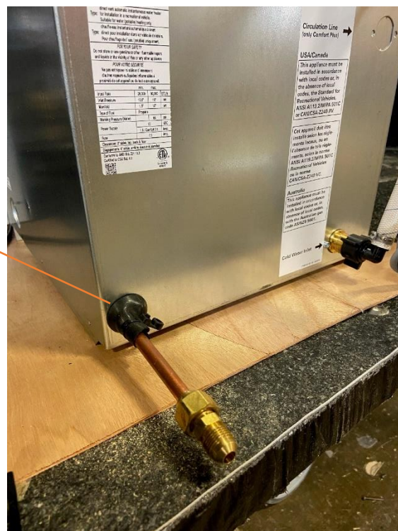
Rear entry gas line viewed from coach side
