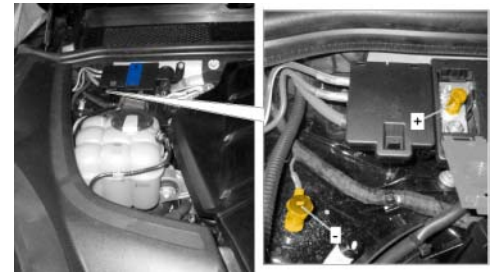
External power connection
