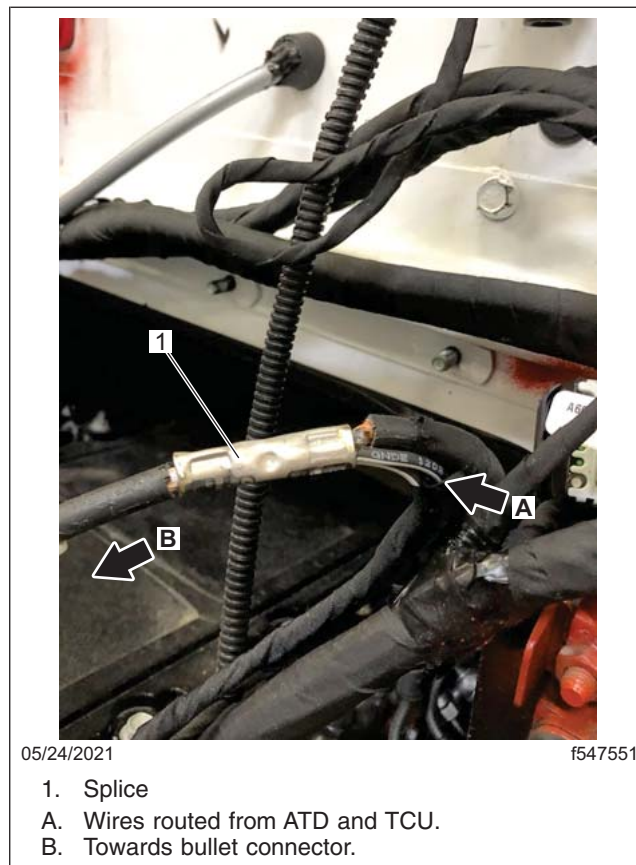
Fig. 11, Overlay Harness A66-13193-011 Spliced
