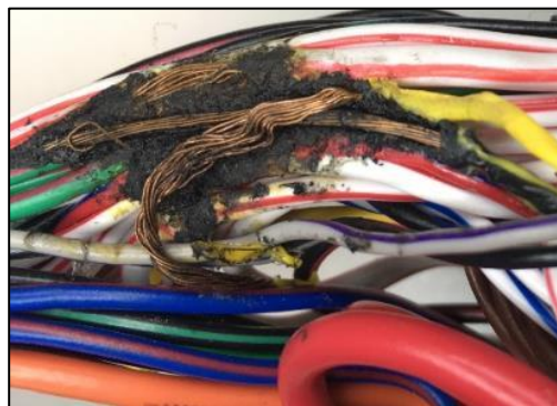
Fig. 6 - Severe Damage (follow code 02)
