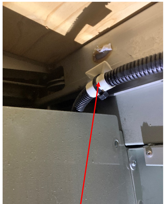
Adhesive base failed. Refer to section 5.3 for rework
