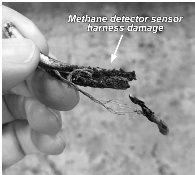
Figure 6, Methane detector sensor harness (damaged).
