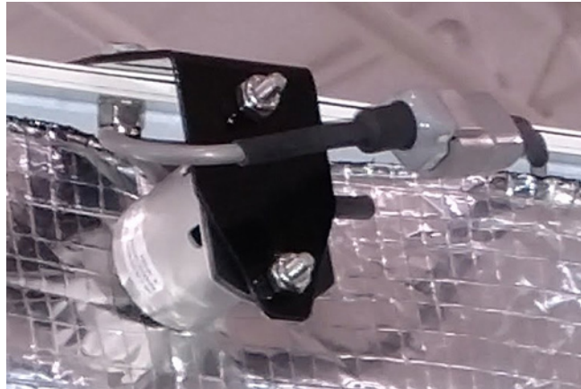
Figure 4, Methane detector sensor harness (undamaged)
