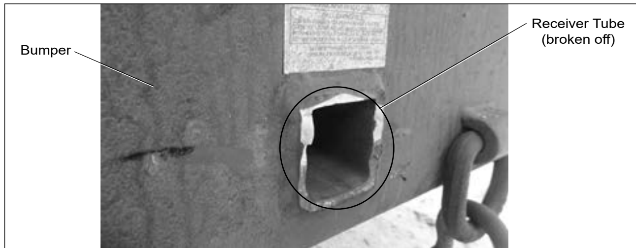
Figure 3 — Structural Failure Example
