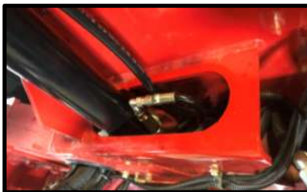
Figure 9 Close-Up of Velocity Fuse Assembly
