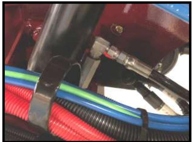
Figure 6 Close-up of Velocity Fuse Assembly
