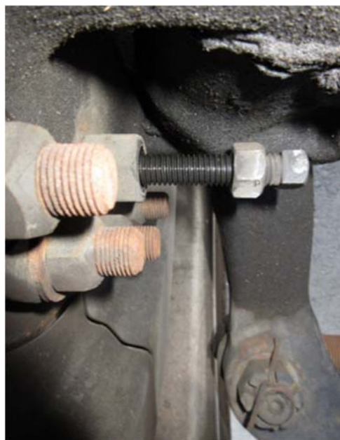
Figure 7 – Loose and Bent Stop Bolt
