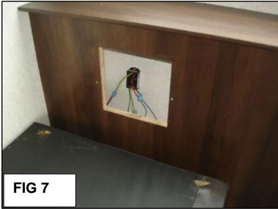
FIG 7: The light control module and wiring are located in the cabinet.
