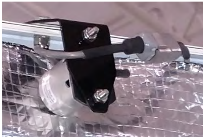
Figure 2, Methane detector sensor harness (undamaged)
