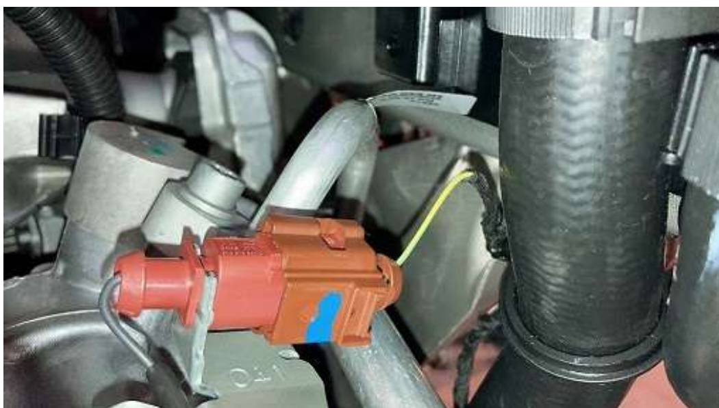
Figure 2. Connector in its repaired state.
