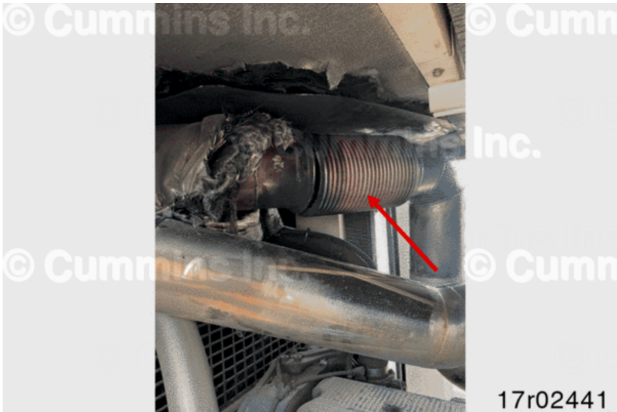
Figure 3, Old-Style Failed Bellow
