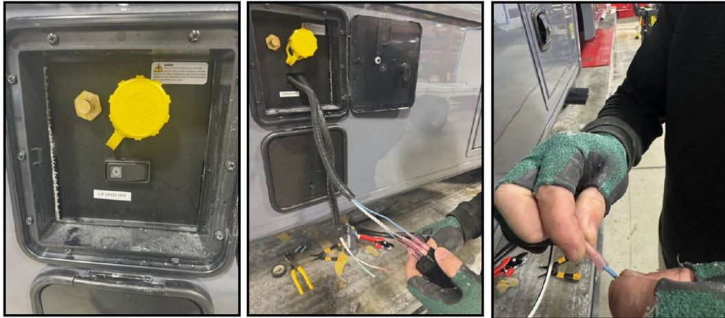
Fig. 3 — LP shut-off switch removed from access panel.
