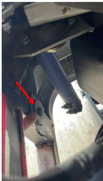
Figure 5: Existing bolt at the RH rear frame
