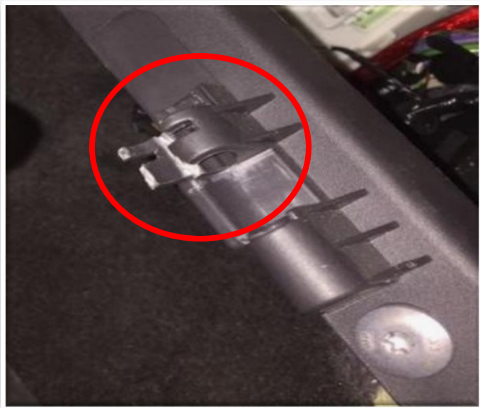
Cracked or broken attachments indicated by white stressed material.
